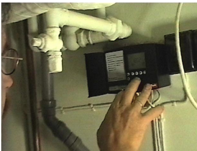
Figure 4: A heating installer confronted with a modern electronic heating controller with display and push buttons. There is no possibility of transferring skills from their work practice.
